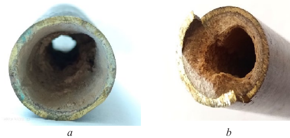
Fig. 1. Photos of a cross section of heat exchange pipes with scale deposits: (a) – condenser pipe, d = 28\text{ mm} ; (b) – peak boiler pipe, d = 19\text{ mm} .
