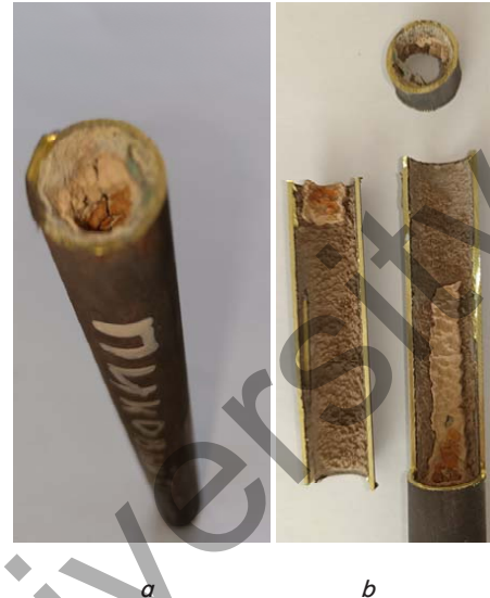
Fig. 3. Peak heat exchanger: a – photo of the scale formed inside the peak boiler; b – images of the peak boiler
