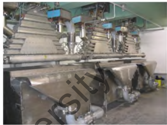
Figure 8. Waste water treatment room in the dyeing center. Daegu, South Korea
