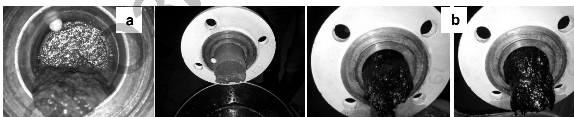
Figure 5. Cleaning of pipe from mechanical impurities and corrosion deposits (a) and from ARPD (b)
