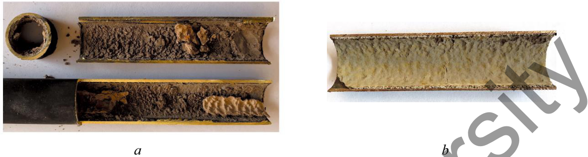
Figure 2. Samples of heat exchange pipes sections from CHPP-3 after operation during the heating season: a) — boiler pipe, d=19\text{mm} ; b) — condenser pipe, d=28\text{mm}
