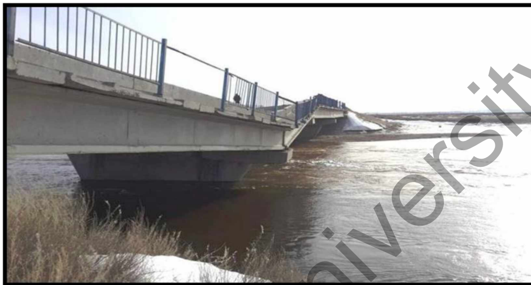
Figure 2. The bridge across the rivers near Sarysu, destroyed by floods [6].
